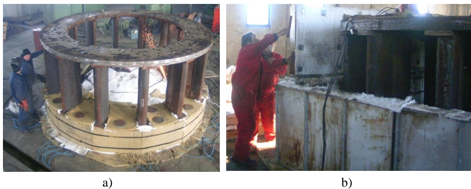
Fig. 5. Equipment for heat treatment during and after repair welding, a) preheating equipment, b) furnace for PWHT.
