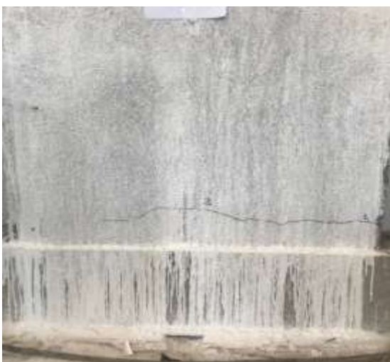
Figure 12: Development of cracks in the RW 1 wall
