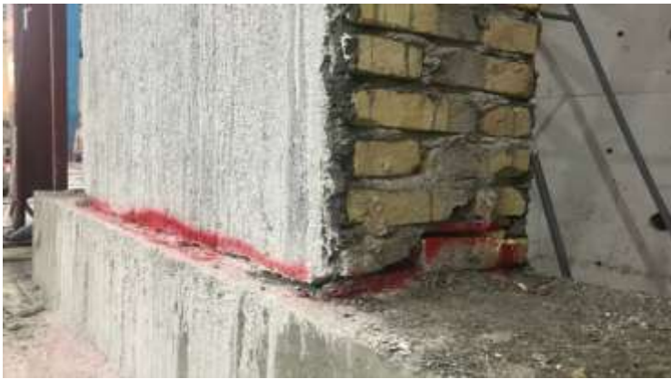
Figure 15: Development of cracks in the RW 2 wall
