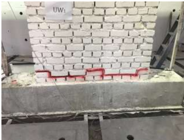
Figure 9: Crack development at a drift
